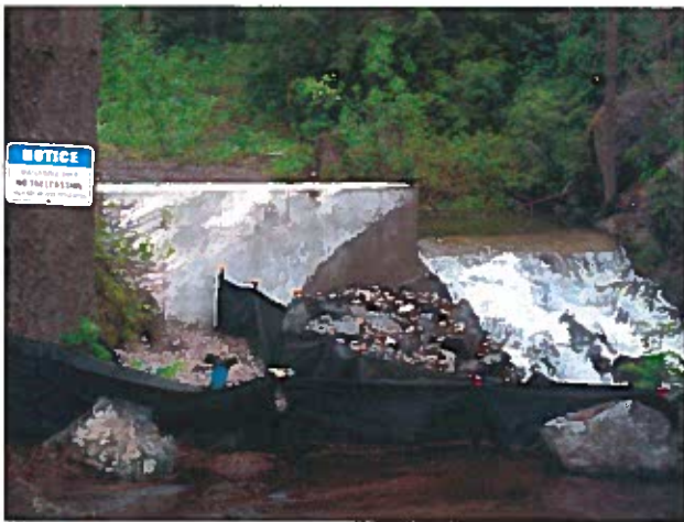
Topping Creek Raw Water Intake
